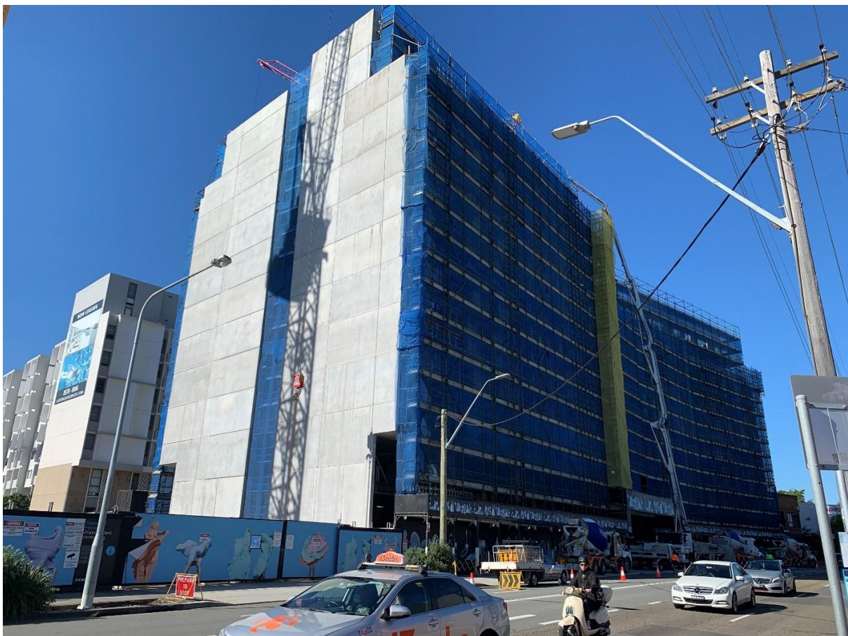
Figure 12: View to Lateral mixed use development site at nos. 501-515 further south on Botany Rd.
