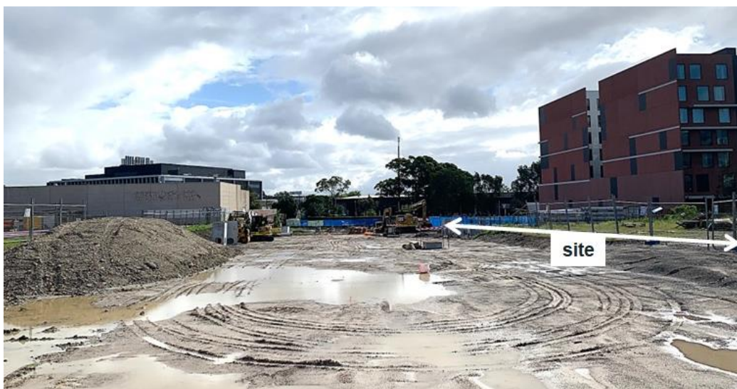
Figure 4: Frontage of subject site to future GS2AC Road and which is currently under construction (viewed from its eastern end, looking west).
